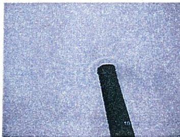
#5 Water Heater Exhaust
